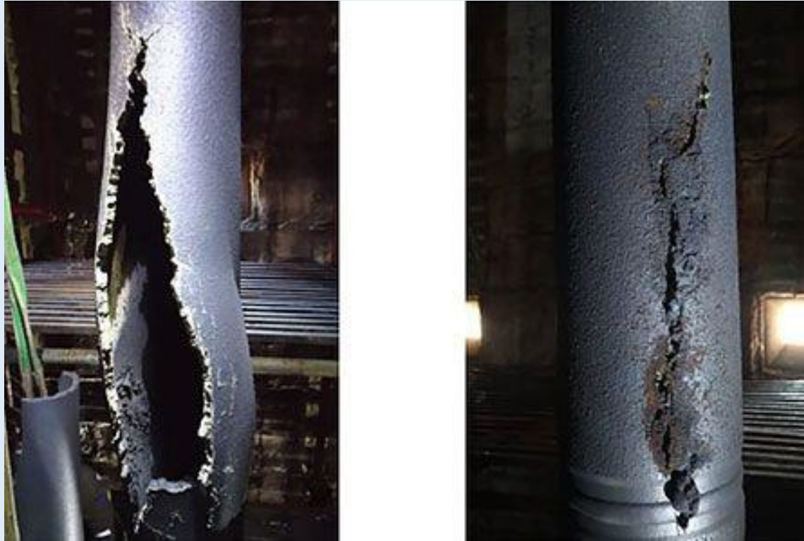
Reformer Tube Failure due to Creep
